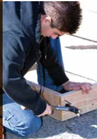
■ Nasi Feles hammers out the frame of a house that will be sent to Mexico.
